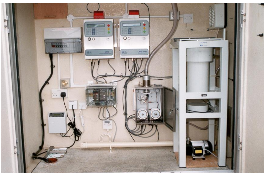
Inside Ramsey Monitoring Station
