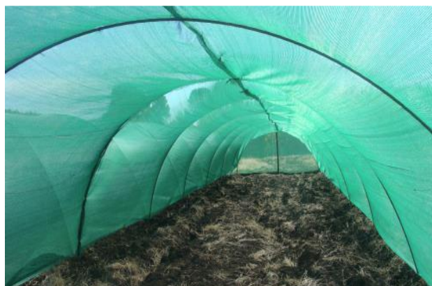
Shade net at Morifi village which was constructed during the reporting period. PHOTO: ActionAid
