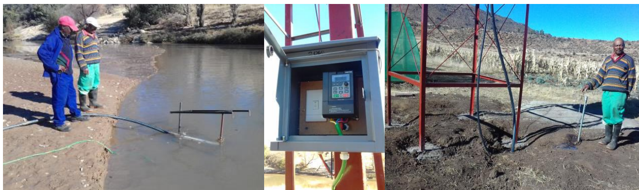
Irrigation scheme at Morifi village pictured at the river, solar pump switch and the tap. PHOTO: ActionAid
