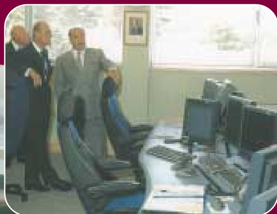
Chairman, John McCallion, Chief Executive Mike Proffitt and HRH Duke of Edinburgh in the Control Room at the CCGT Pulrose Plant.
