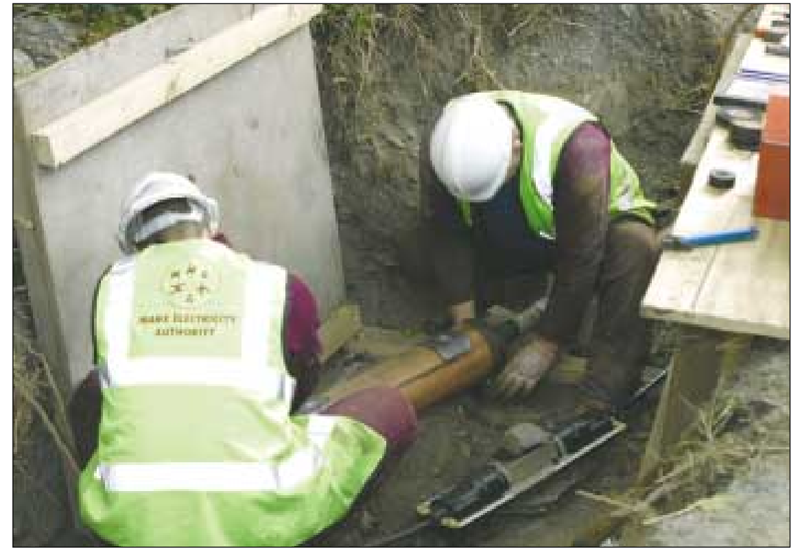
Network Services underground cable jointing team completing a high voltage cable joint on a 11,000 volt cable recently installed under the Sulby river.
