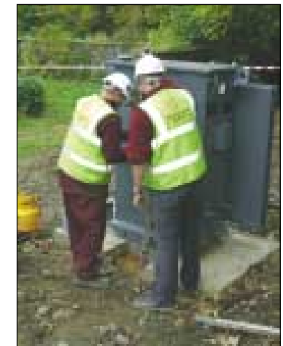
Network Services underground cable jointing team preparing to terminate a low voltage cable to a distribution transformer to facilitate works in connection with the upgrade of the Sulby water treatment plant.
