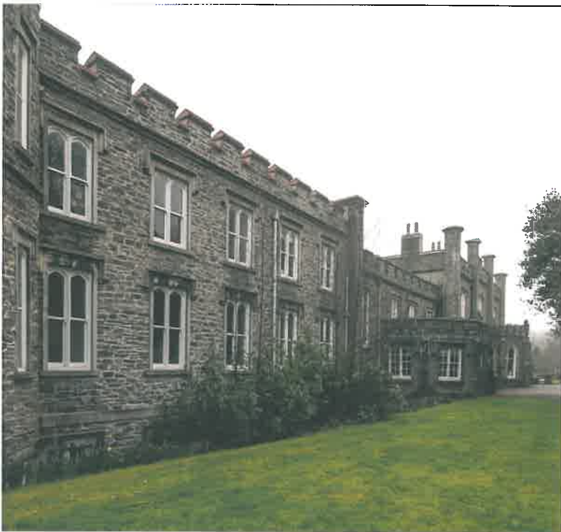
North elevation: phases two, three and four, up to and including the first projecting bay. Windows have hood mouldings above rendered bands to the jambs and heads, and rendered cills. A string course separated the first floor from the parapet. The red ceramic (?) copings to phase four (nearest) are discordant. The basement window-frames are in poor condition. The stonework has been repointed. PAT/6.4.2015
