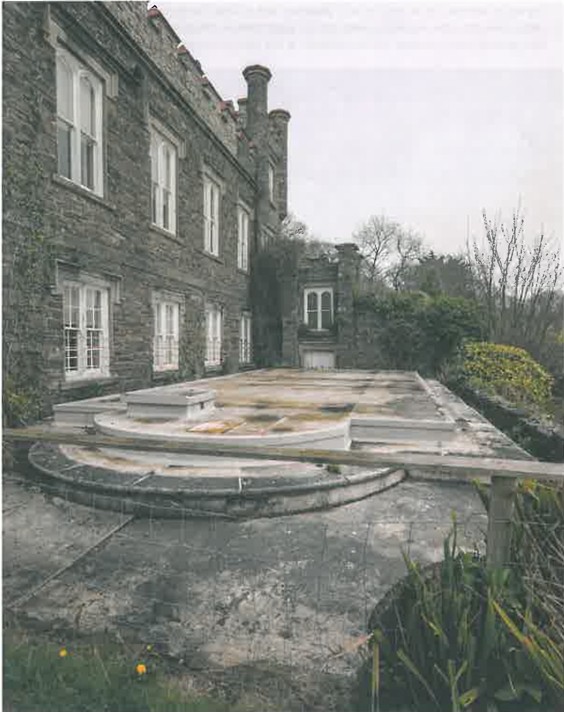
The site of the former swimming pool, which is covered over. Adjoining windows are barred, to prevent accidents. PAT/6.4.2015
