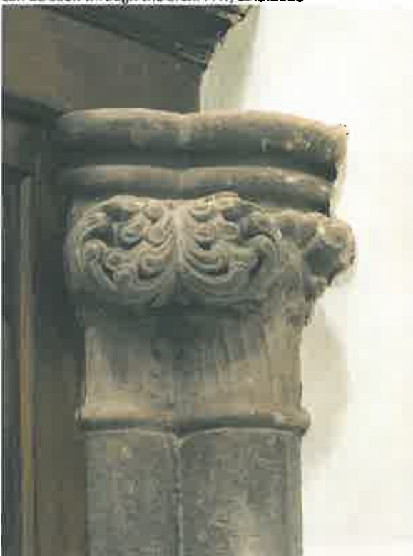
Bundled column with Romanesque capitals are built into the chapel rood screen. They may be the remains of the chapel cloister as described by several writers. Note the oak leaf above the lower annular ring. PAT/9.4.2015
