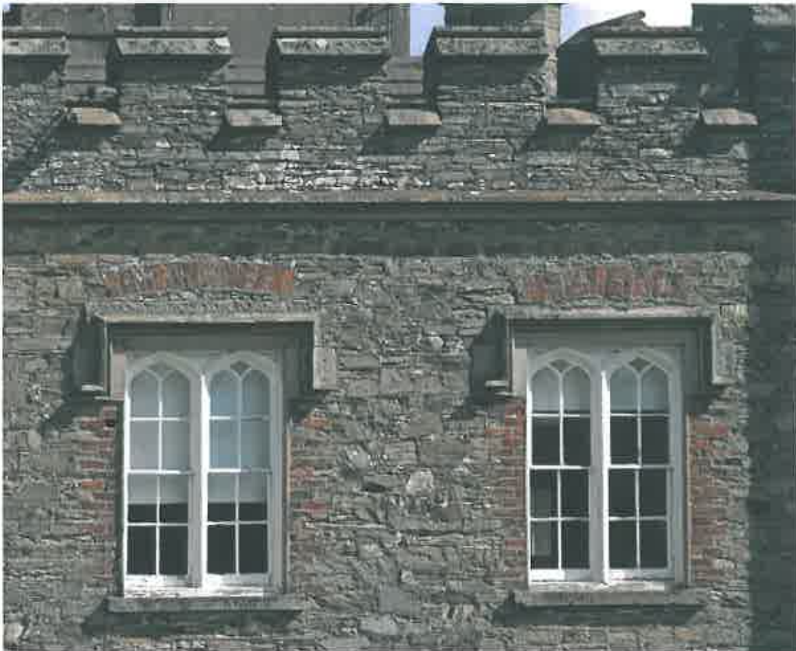
Window details showing the use of engineering brick. Note also the different colour of the stone in the parapet. Pat/12.4.2015
