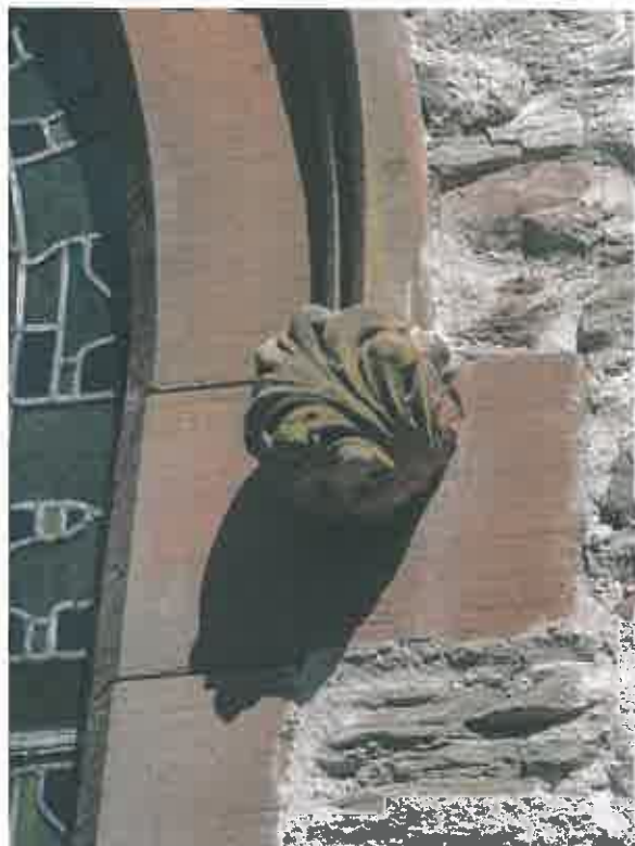
Sandstone label stop to Chapel chancel side window. Similar stops are on the window in the east elevation of the Stable Building. PAT/7.4.2015
