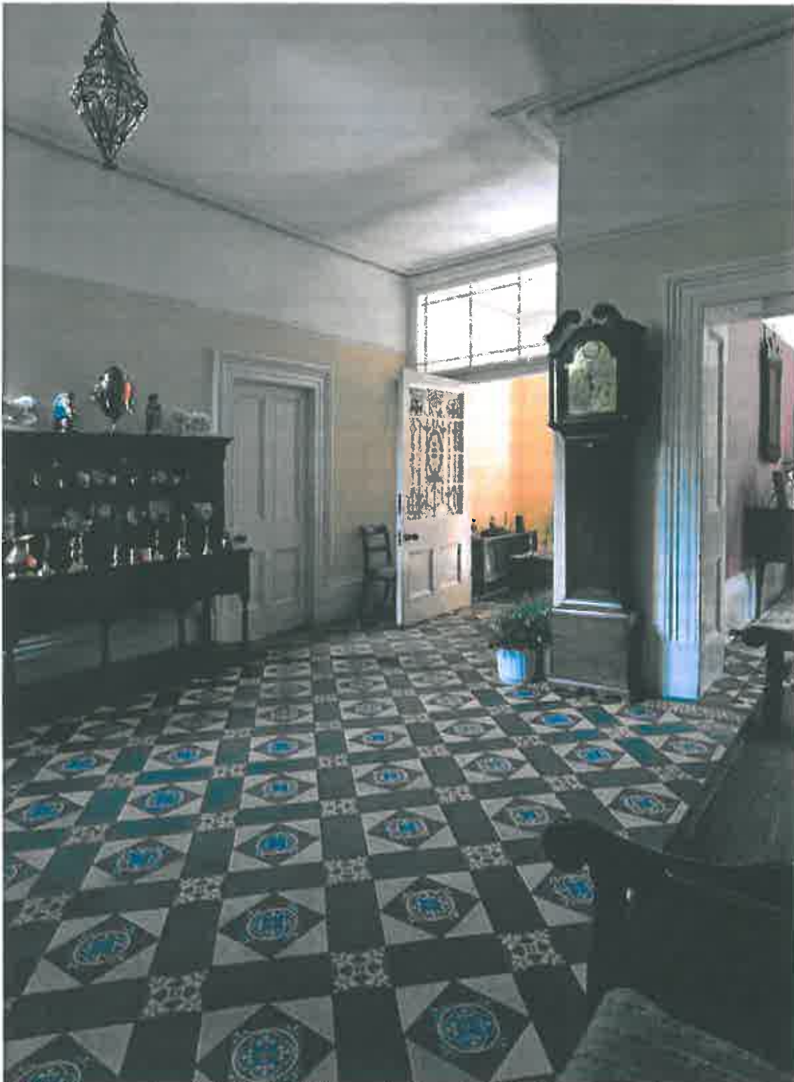
Hall, looking towards vestibule. The inlaid tiles may date from the 1840s. They are normally protected under carpets. The floor is entire and in excellent condition. The tea urn on the dresser was used in Tynwald Mills. The vestibule screen has Georgian elements (the proportion of the clerestory lights and the columnettes (not visible in this view) but the stained glass appears of a later date, probably Victorian or Edwardian. Note also the size and depth of the architraves and skirtings.
