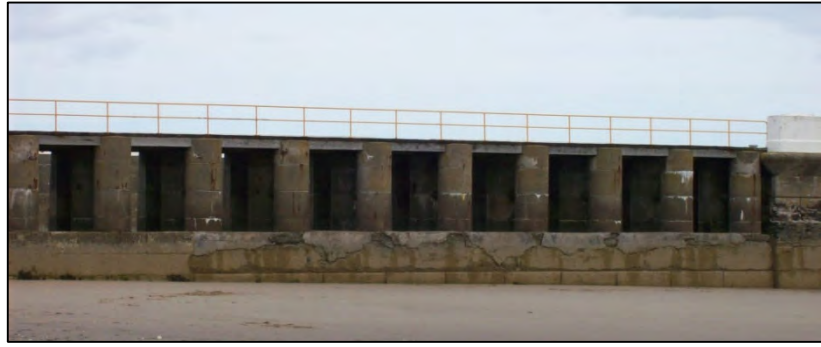
Photo 8 – Openings in South Pier
