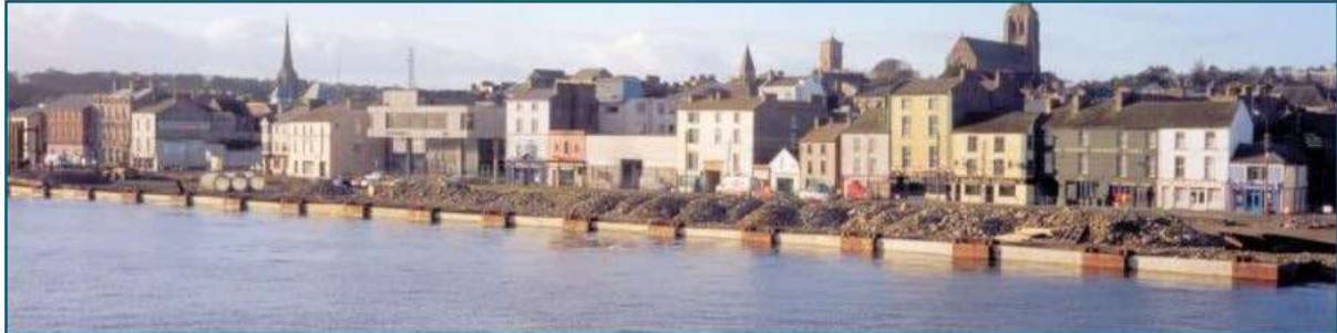
Figure 17: Wexford in the Republic of Ireland - New Fisherman's Quay - Caisson Wall Construction
