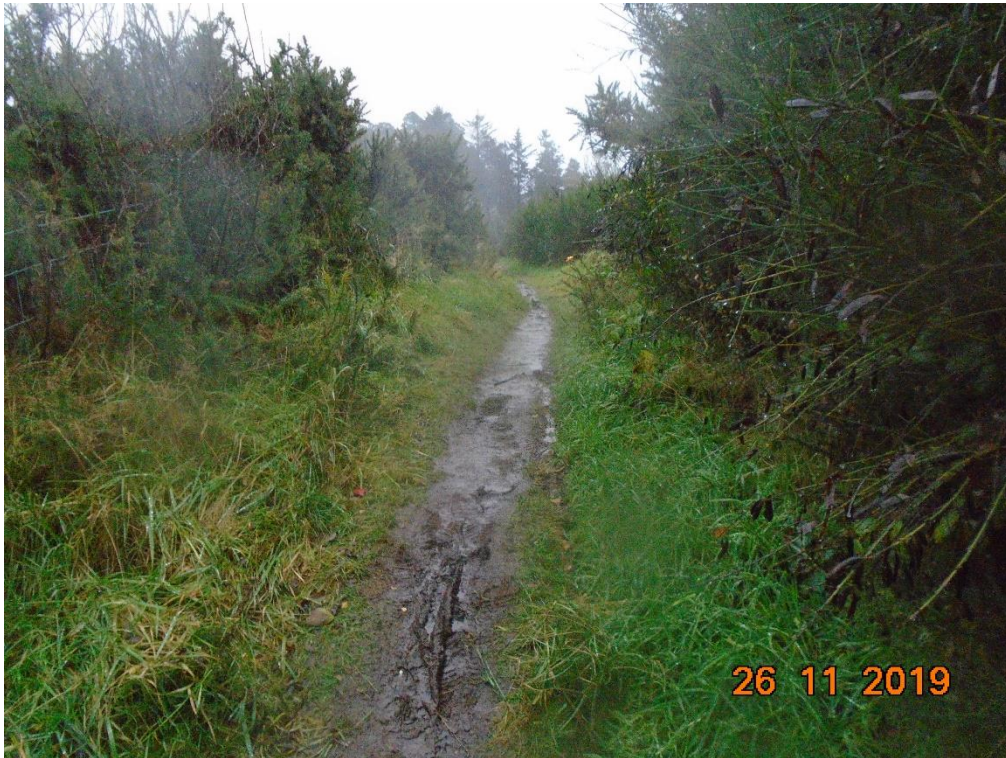
Photograph 3: Crest of western embankment. Fence and downstream slope on left of photo.
