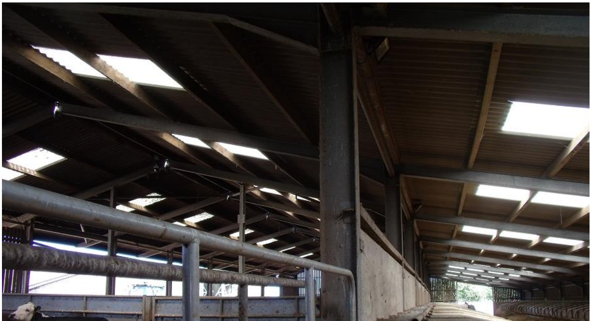
Figure 3: This shows a lean-to extension that leads onto an open ventilated ridge from the inside.
