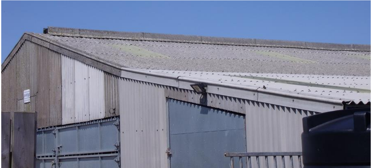
Figure 2: This shows a lean-to extension that leads onto an open ventilated ridge.
