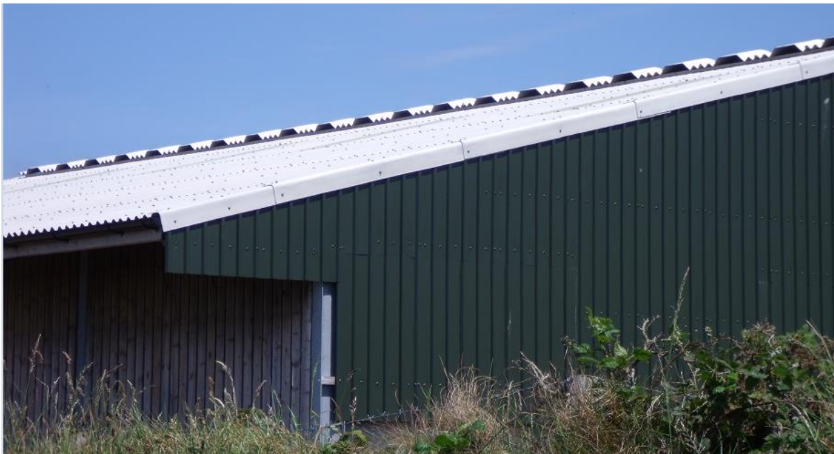
Figure 1. This is showing a normal crown crank ridge raised up on a 25mm wooden baton.
