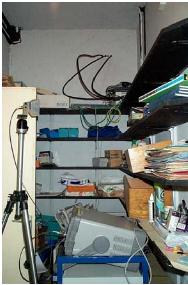
Picture 7 Microwave signal generator and feeder cables in the Storeroom
