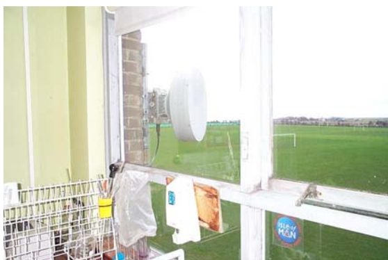
Picture 6 26 GHz microwave dish outside the Preparation Room
