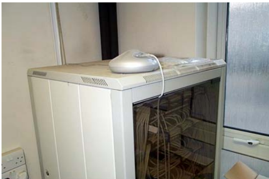
patch panel cabinet
