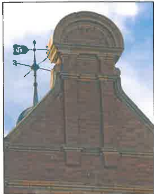
Pilasters support the entablature of the decorative arched capping to the gable. This and the steep-sided nature of the gable contribute a Flemish element to the
