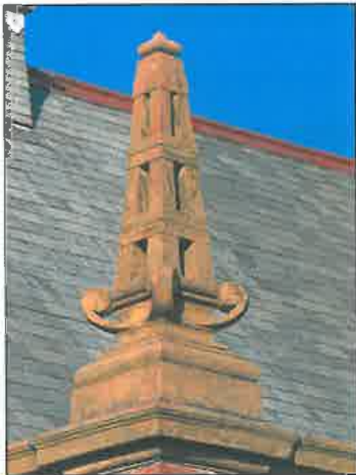
Pinnacle, north-east corner. Enlargement. Note the detail and finish which gives the impression of a sandstone sculpture.
