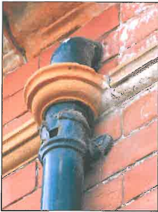
Unusual terracotta moulding feature around down-spout. Note progressive degradation of surface
