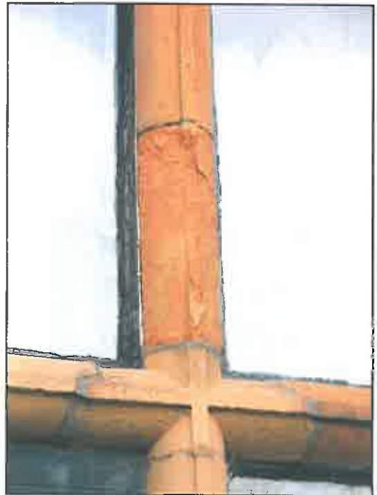
Transom and mullion terracotta sections. Note progressive degradation of surface
