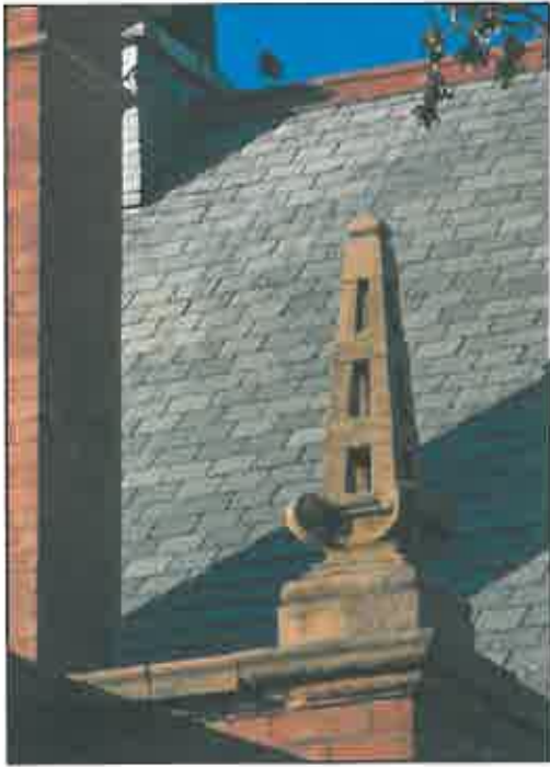
Pinnacle, north-east corner. Note the good colour and condition of the green Welsh slate.
